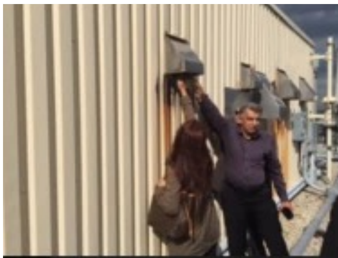
Ambient temperature coming from the boiler flue gas. Those in attendance put their hands in the 84.6F flue gas exhaust while the boilers were operating.
