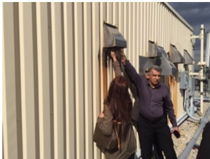
Ambient temperature coming from the boiler flue gas. Those in attendance put their hands in the 84.6F flue gas exhaust while the boilers were operating.
